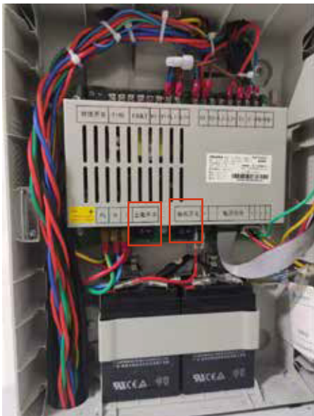
Internal View of Fire Protection System Control Box
