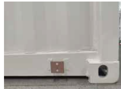
— Grounding Wire Location
